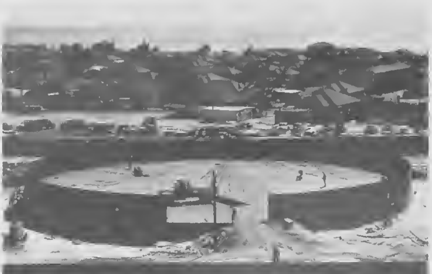
5 THE WALLS start up. From here, building tanks is like putting together a puzzle; every piece of steel has its place. E MURAYANAN ta cuminza bai laria. For di aki, trahamento di tanki ta manera trahamento di un rompecabeza.
